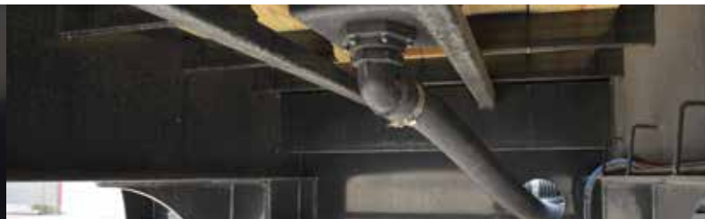
All Plumbing Under the Deck
