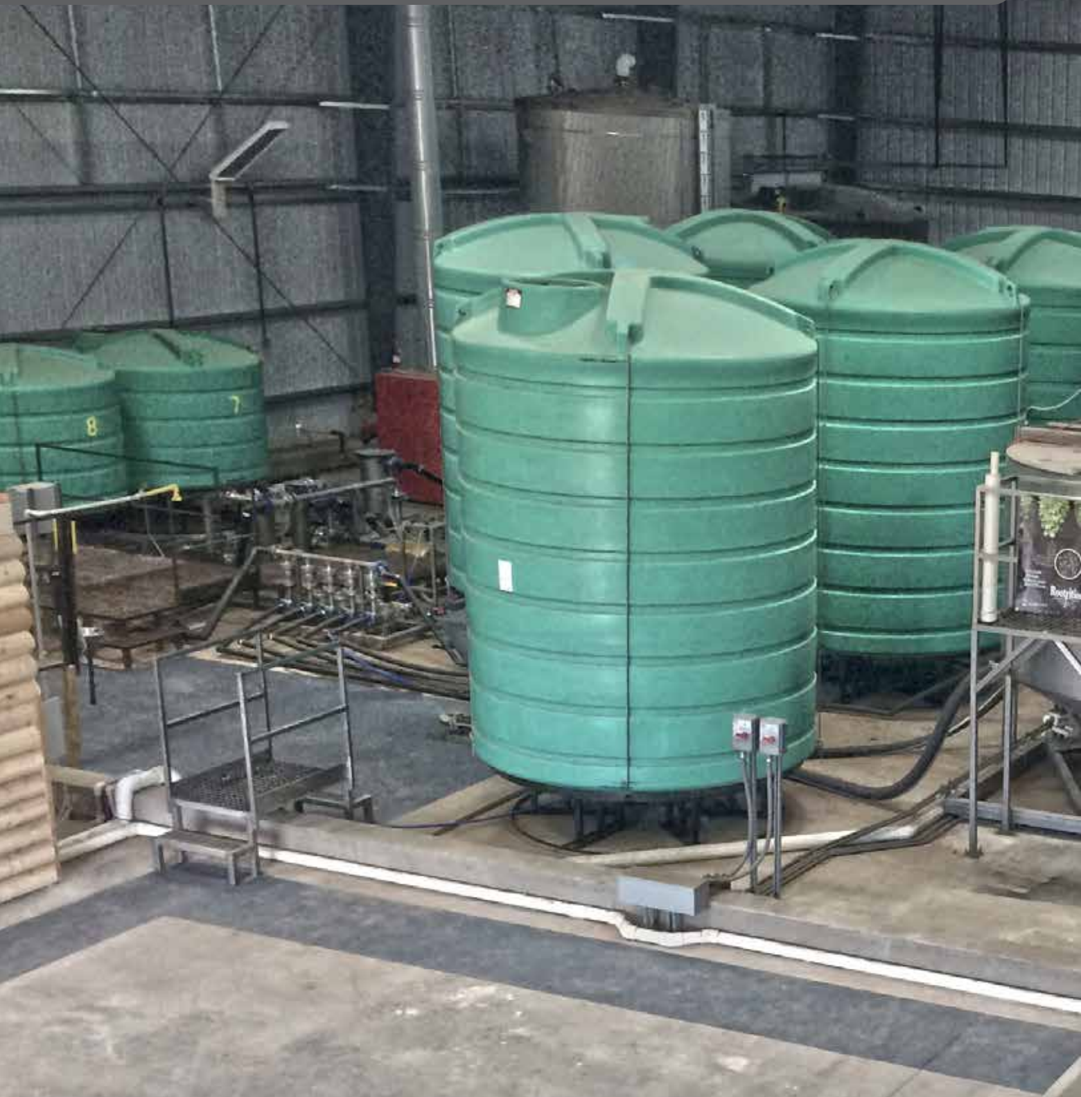
Featured Image: 5,000 Gallon Cone Bottom Storage Tanks (THC05000K)
